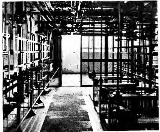
FIG. 8.—REAR OF SWITCHBOARD IN POWER HOUSE.
